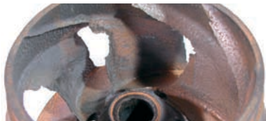
Erosion corrosion of cast iron impeller
